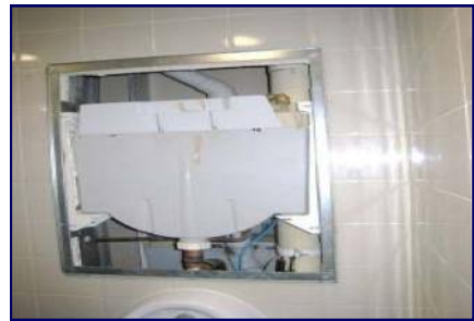
Typical in wall cistern installation before installation of solenoid valve
