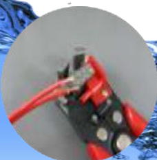
Cut and stripe the cable.
